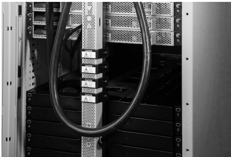
Figure 10.5 – Rack bus bar
